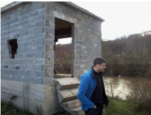
Destroyed hydrometric station at river Drin (near Kralan)
